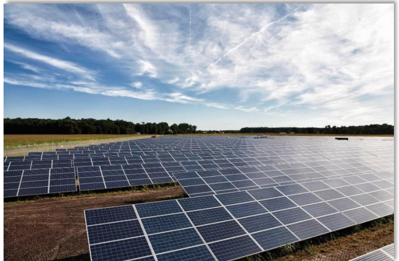
The first phase of the Bruce A. Henry Solar Farm became operational in 2013.
