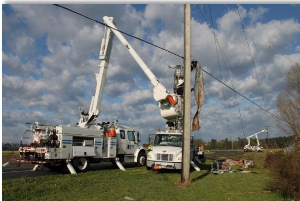
Delaware Electric Co-op crews restore power to affected members after an April 15 tornado passed through the service territory.
