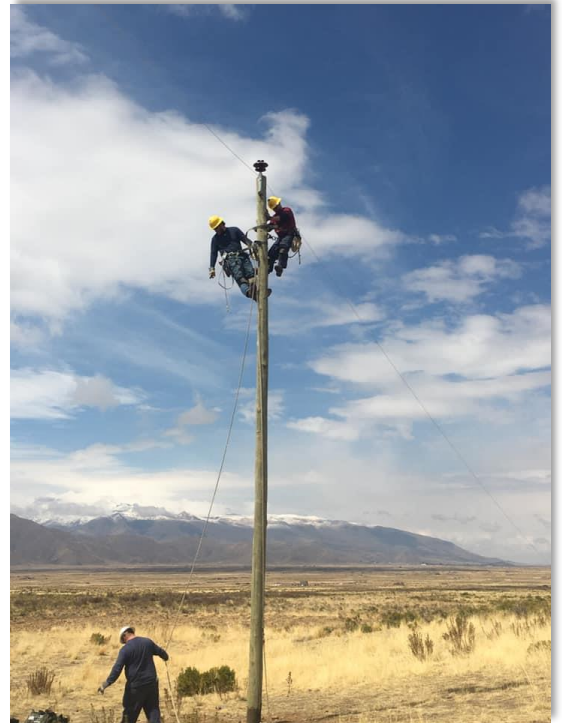
With snow-capped mountain peaks as a backdrop, VMD crews string wire that will bring power for the first time to several rural Bolivian villages.
