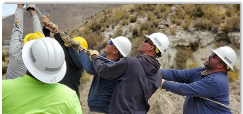
Several lineworkers team up "old-school style" to string wire and bring power to Bolivia.
