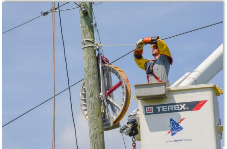
Rappahannock Electric Cooperative has announced a $30 million investment in its fiber network to improve communications and modernize the grid.
