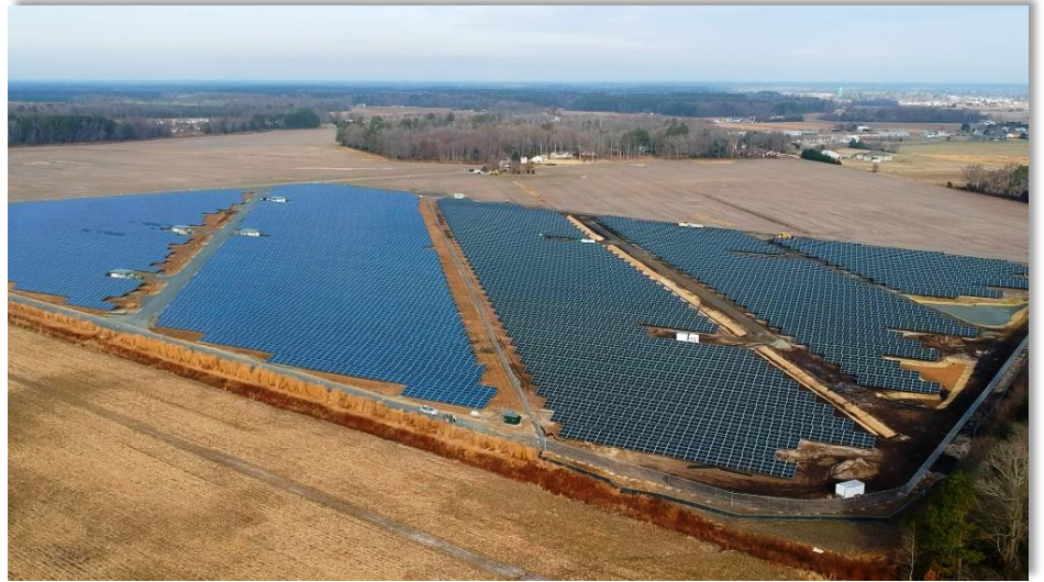
New solar panel arrays have come online at Delaware Electric Cooperative's Bruce A. Henry Solar Farm in Sussex County.
